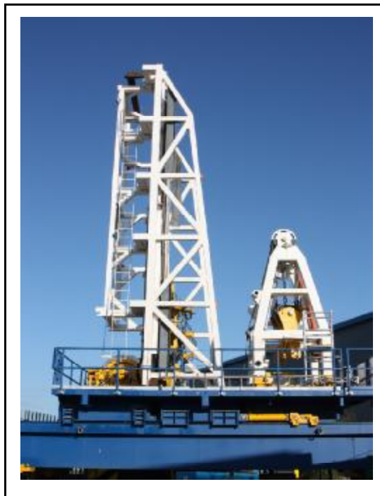
Crown on Cross Travel Carriage. (Lift Trolley Drive Frame & Winch in Place)
