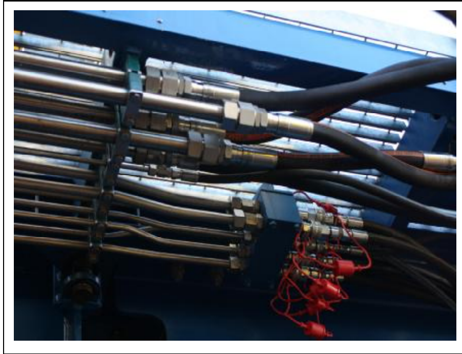
Main Pipework from Control Console
