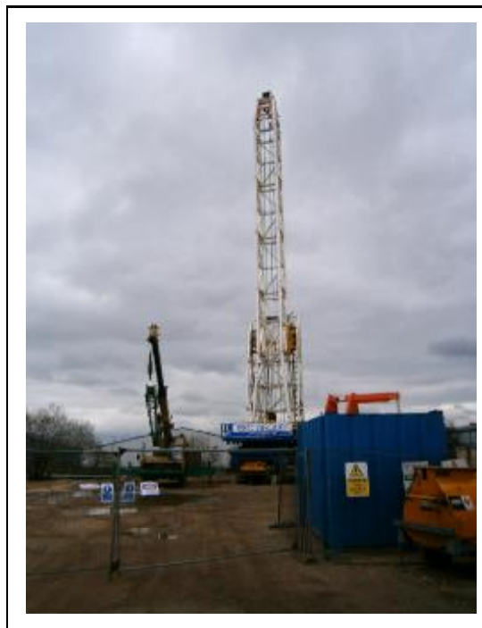
Entire Rig Assembly
