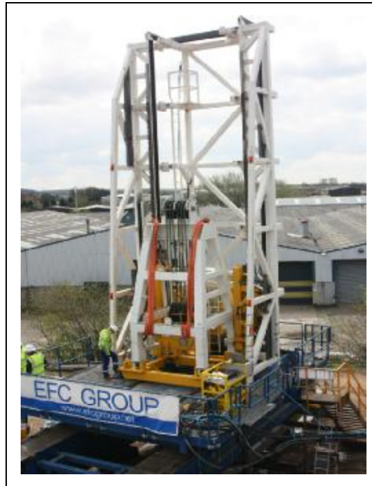
Crown Attached to Lift Trolley
